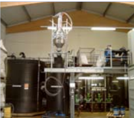
Conveying of activated carbon and other chemicals for waste water treatment. Vacuum Conveyor with electric powered Vacuum Pump.
