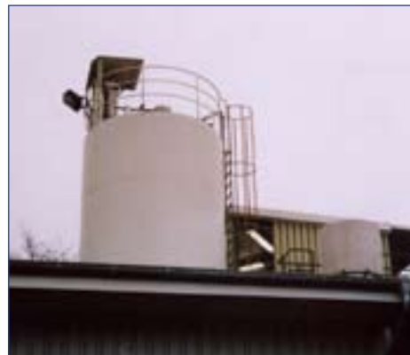
Loading of a silo with iron sulphate powder. 5000 kg/h with VR450, 40 m overall distance, 15 m height.
