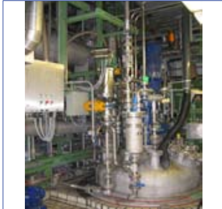
Loading of a reactor with a Pressure Rated INEX (Inert) Vacuum Conveying System. Discharging into an EX zone 0.
