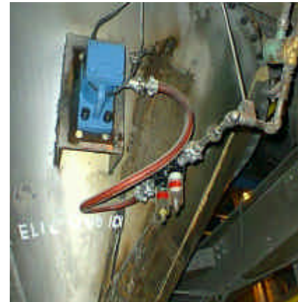
BH installation close-up showing airline accessories
