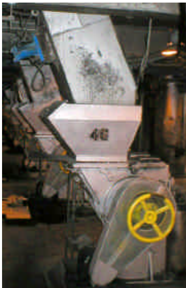
BH on a coal bunker
